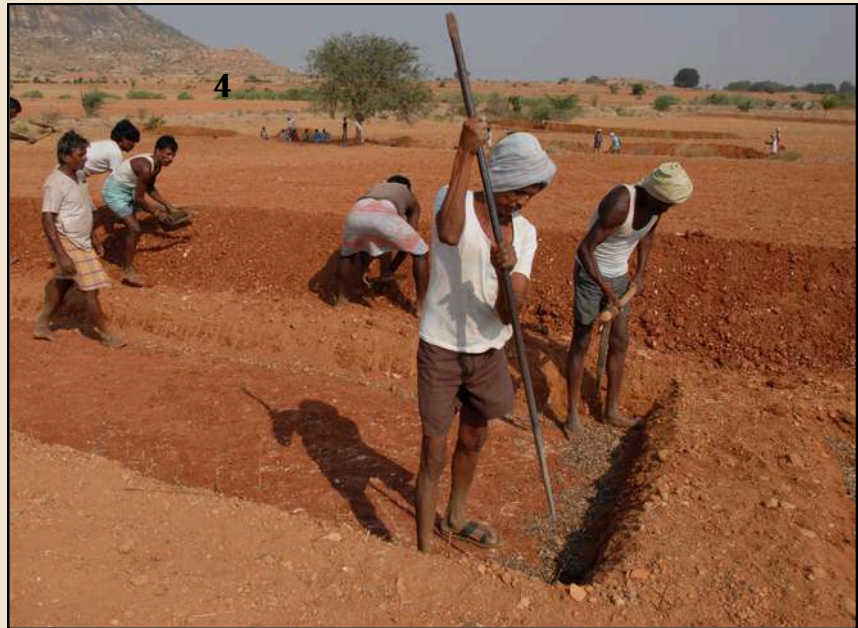
Trenching work in progress at Kundurpi in the early years of Watershed Project implemented by the AF-EC.
